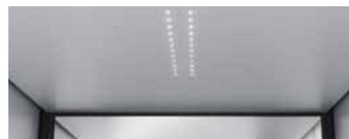
SHAFT CEILING WITH LED LIGHT Energy-saving and durable lighting
